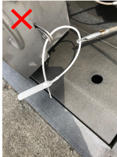
Seal not tightened
